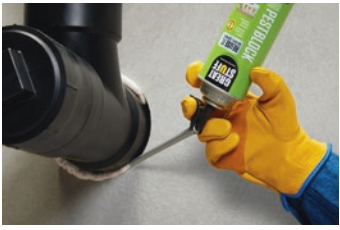
PVC Pipe Penetration
