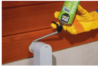
Electrical Cable Lines
