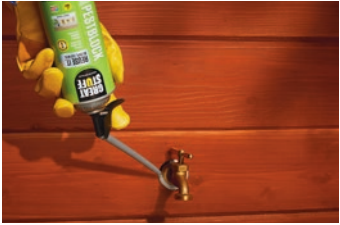
Water Faucet Penetration
